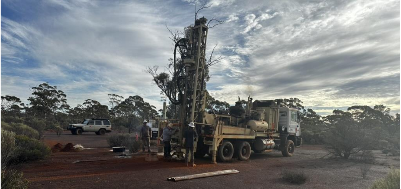
Figure 3: Australian Aircore Drilling AC rig on site at the Northern Zone Project
